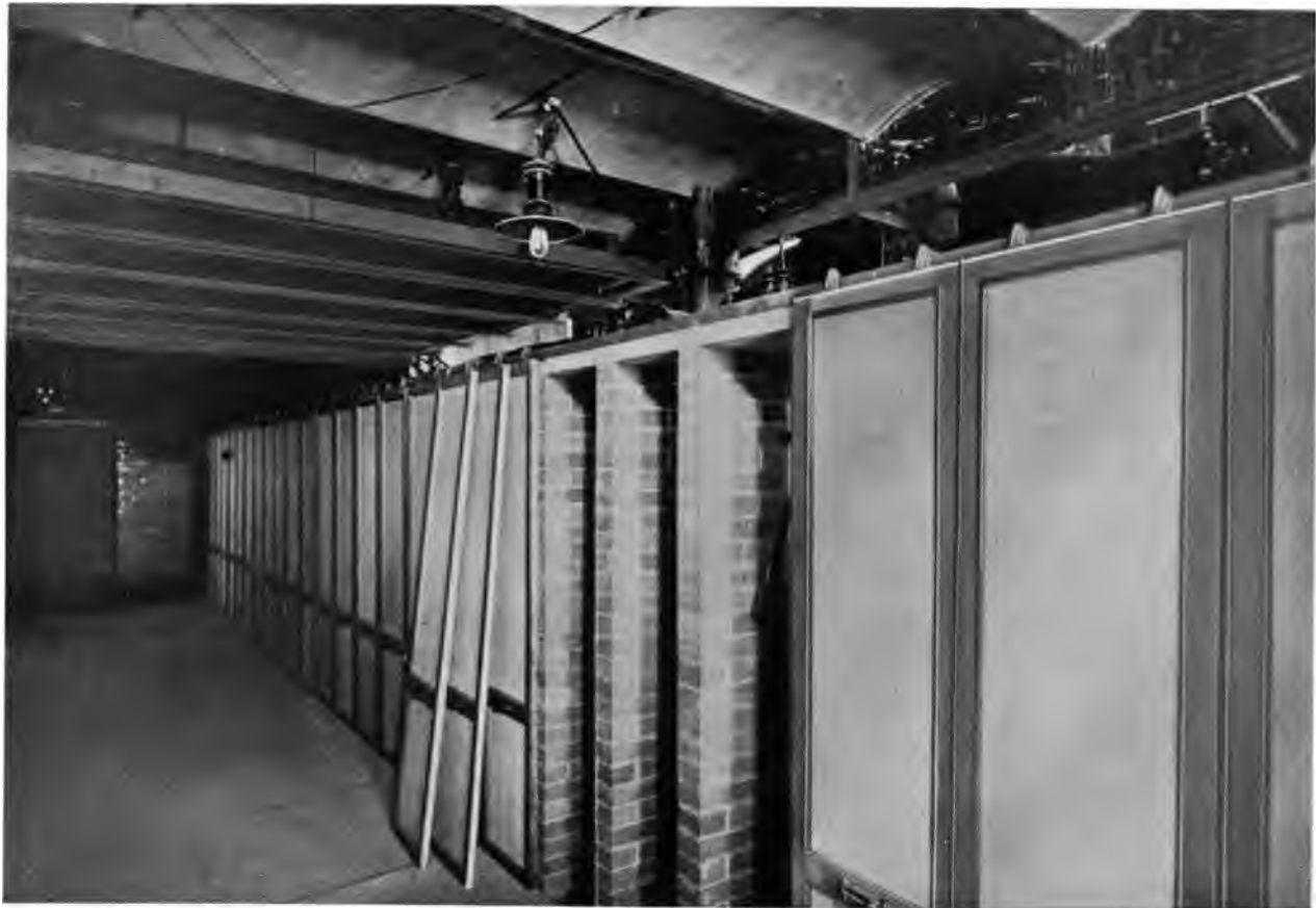
REAR VIEW OF BUS BAR COMPARTMENTS—MAIN POWER STATION
